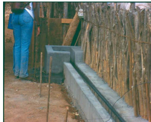
Figure 72: Concrete trough 10cms wide and somewhat high to prevent the young from falling in, the float valve is protected in the background.
