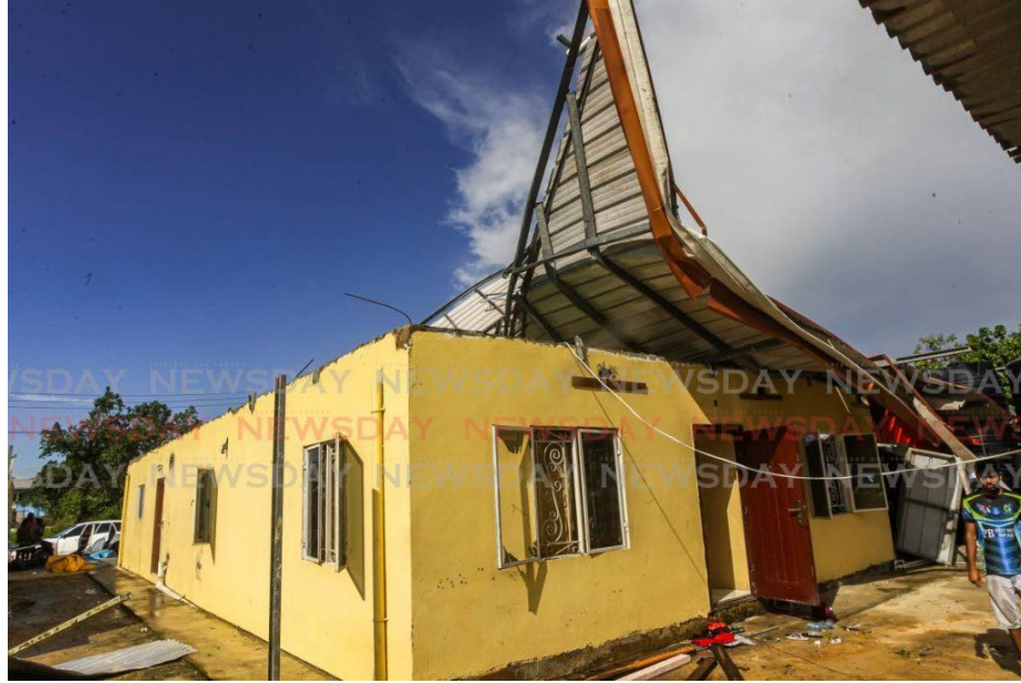
Photo 3: Roof partially blown off in Chase Village Trinidad
