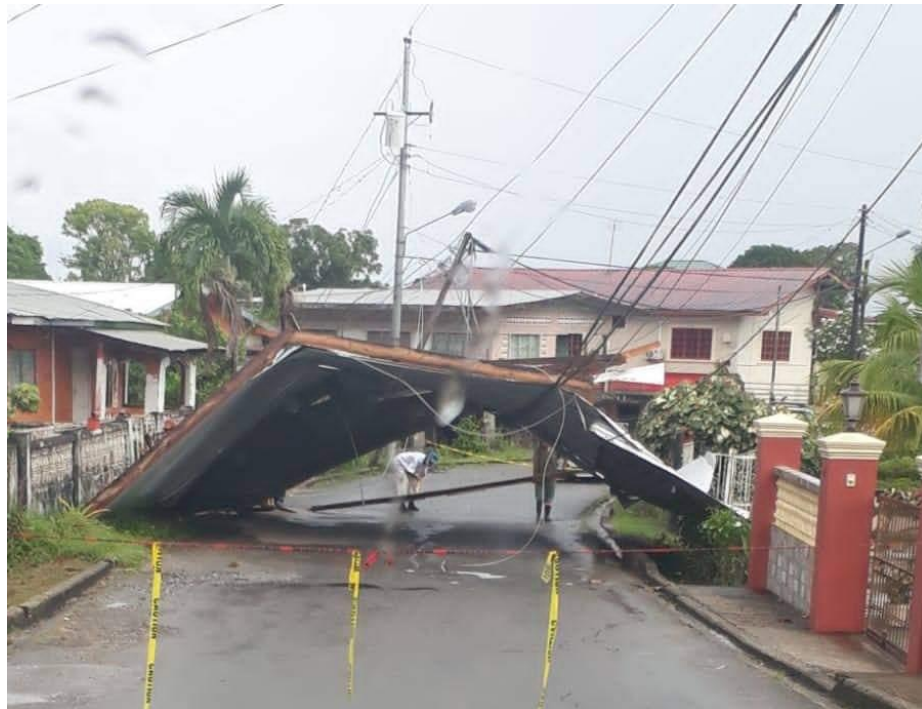
Photo 2: Entire roof blown off in Point Fortin Trinidad
