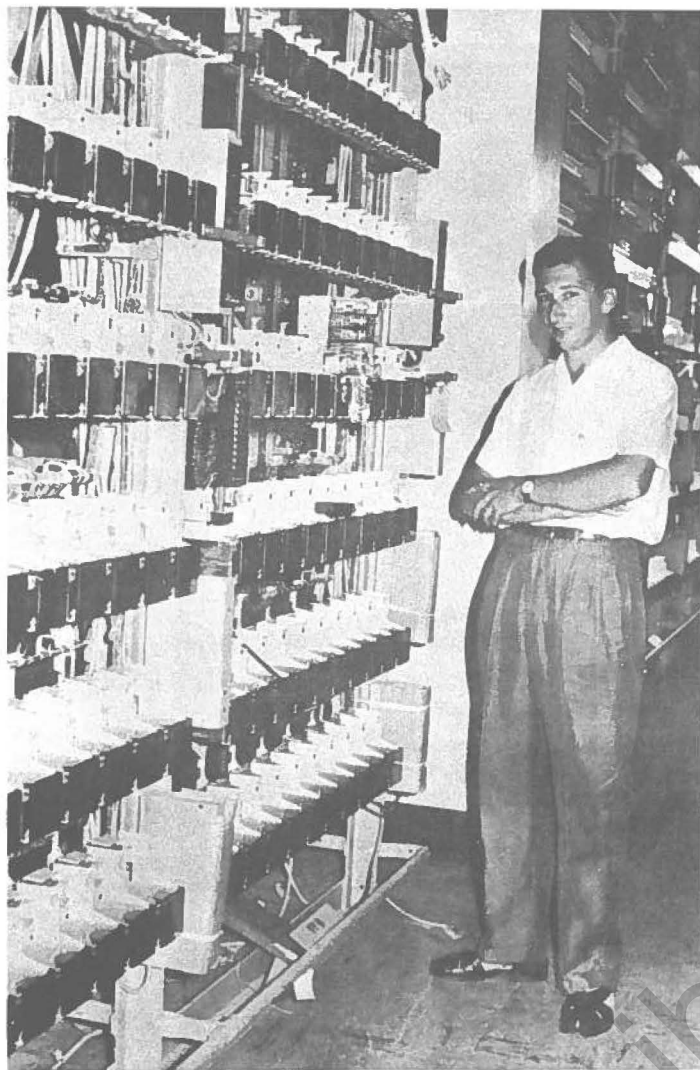
General Electric Engineer G. B. Scott, standing near a rack with some 2,000 selector switches. As chief installing engineer, just out from Bagdad in Iraq, where a similar system was installed, he is now directing the installation by local technicians.
