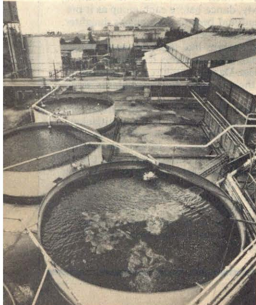
Vaal Reefs uranium processing plant
