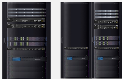
Micro Data Center
