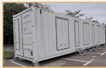
Container Data Center
