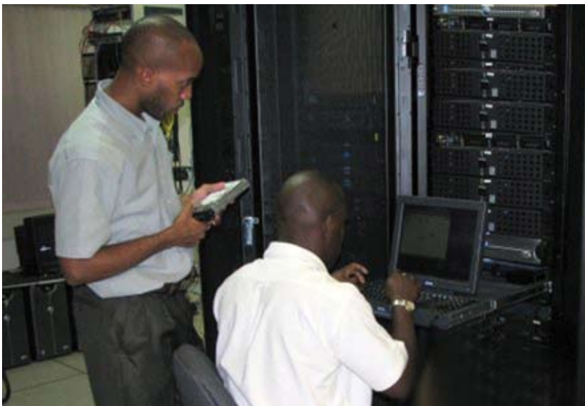
Server Room on Cave Hill Campus
