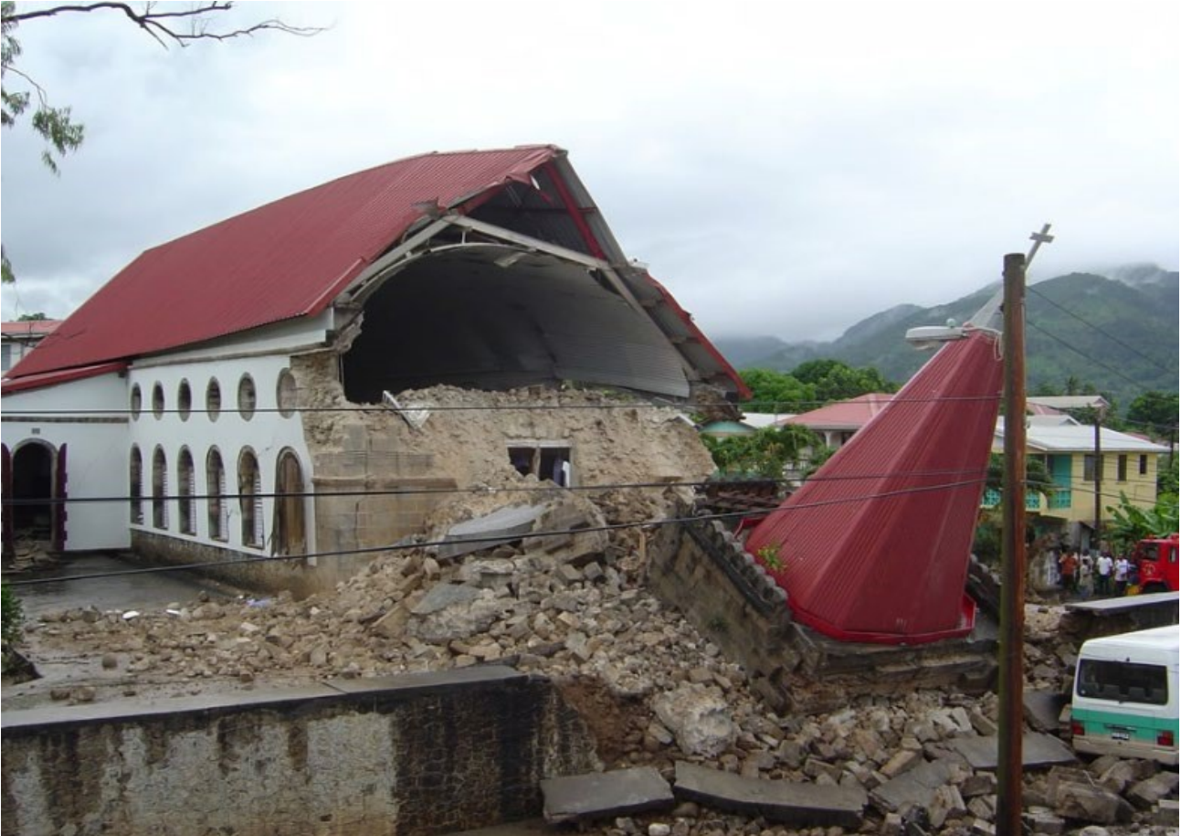
Photo taken after November 21, 2004, earthquake.
