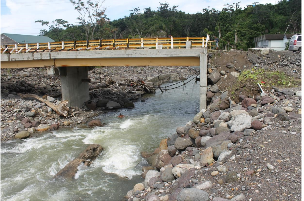
Views of damage to King George V bridge
