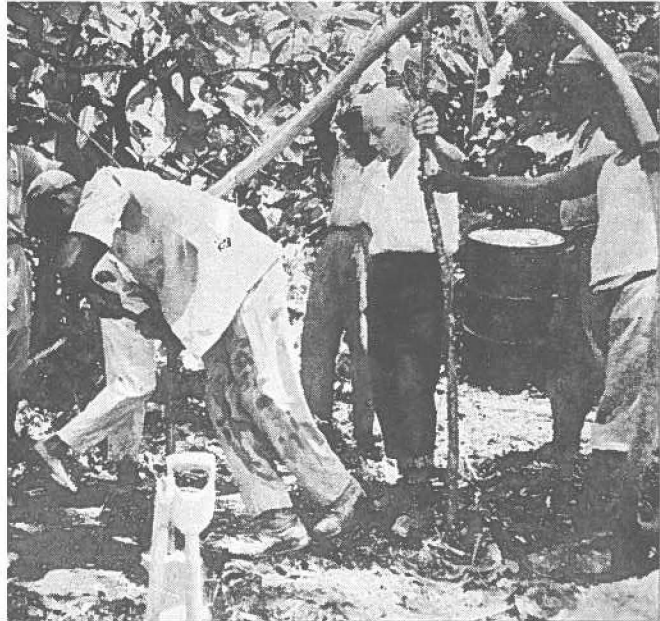
Drilling a shot hole by hand. Note pressure hose supplying water for the operation.
