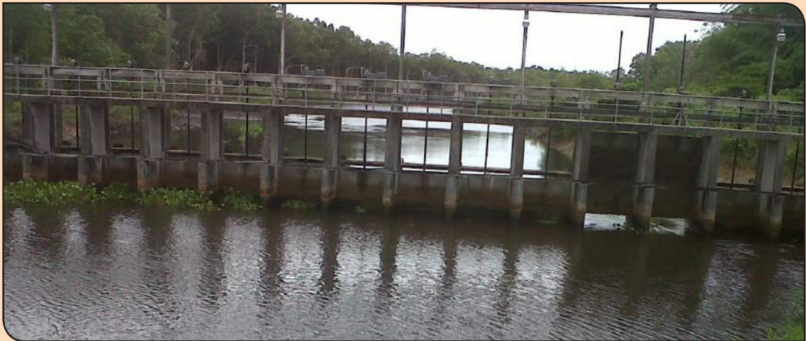
Sluice gate in South Trinidad
