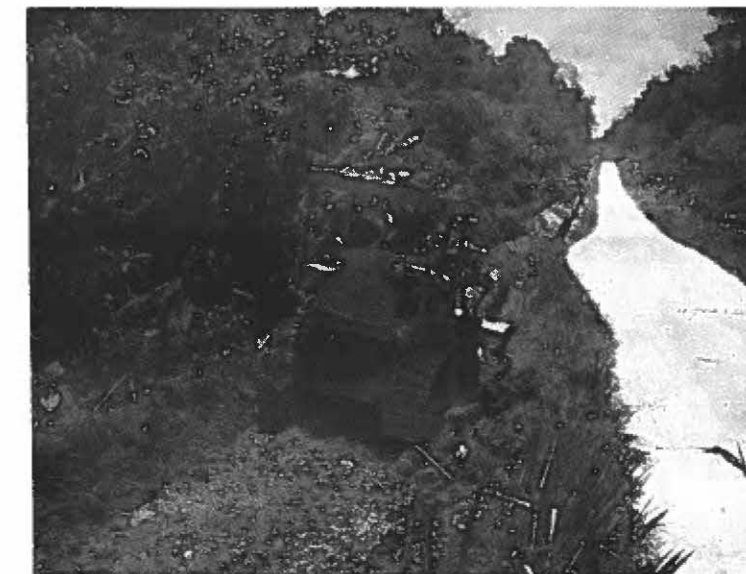
Below, an overhead welder at work on a section of the pipe. Altogether, more than 5,500 welds were made on this line.
