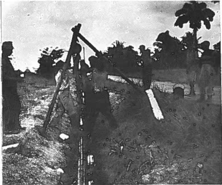
Above, tripod and camel hair belt being used to lower the line. Below, a completed section of the pipeline ready to be buried.
