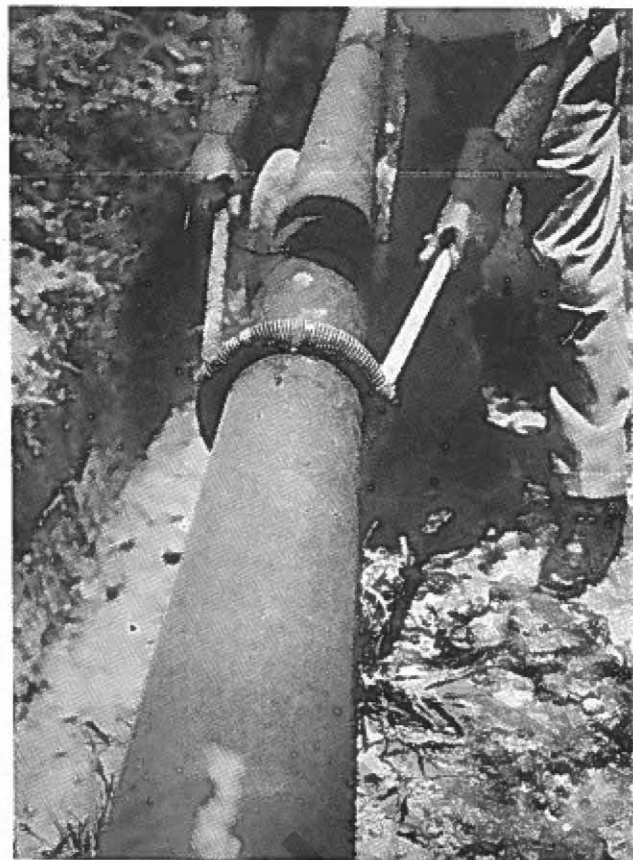
The electrified collar of the Holiday Detector is moved along the hardened bitumen in a search for leaks.
