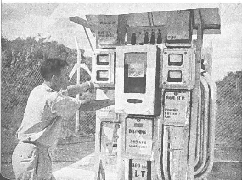
Mr. J. B. Sutherland at a Transformer Station.
