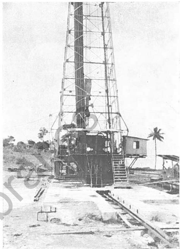
End view of foundation. The rig is skidded 6' 6" towards the camera as each well is completed.
