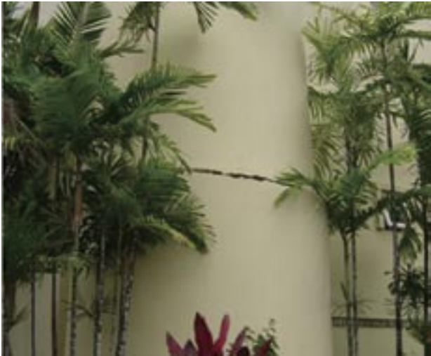
Damage to a building in Trinidad following the 29 September 2006 earthquake.
